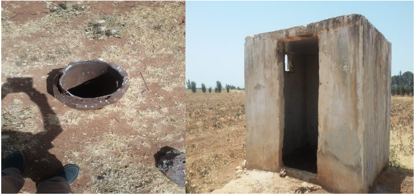
Figure 11: Umahat Al Yadudah groundwater well
