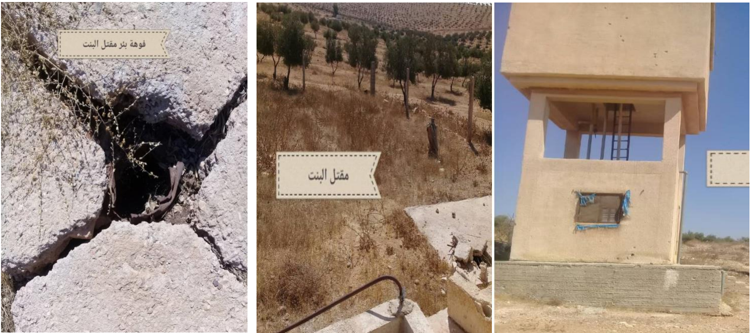
Figure 9: Mktal albint groundwater well -Al Badia
