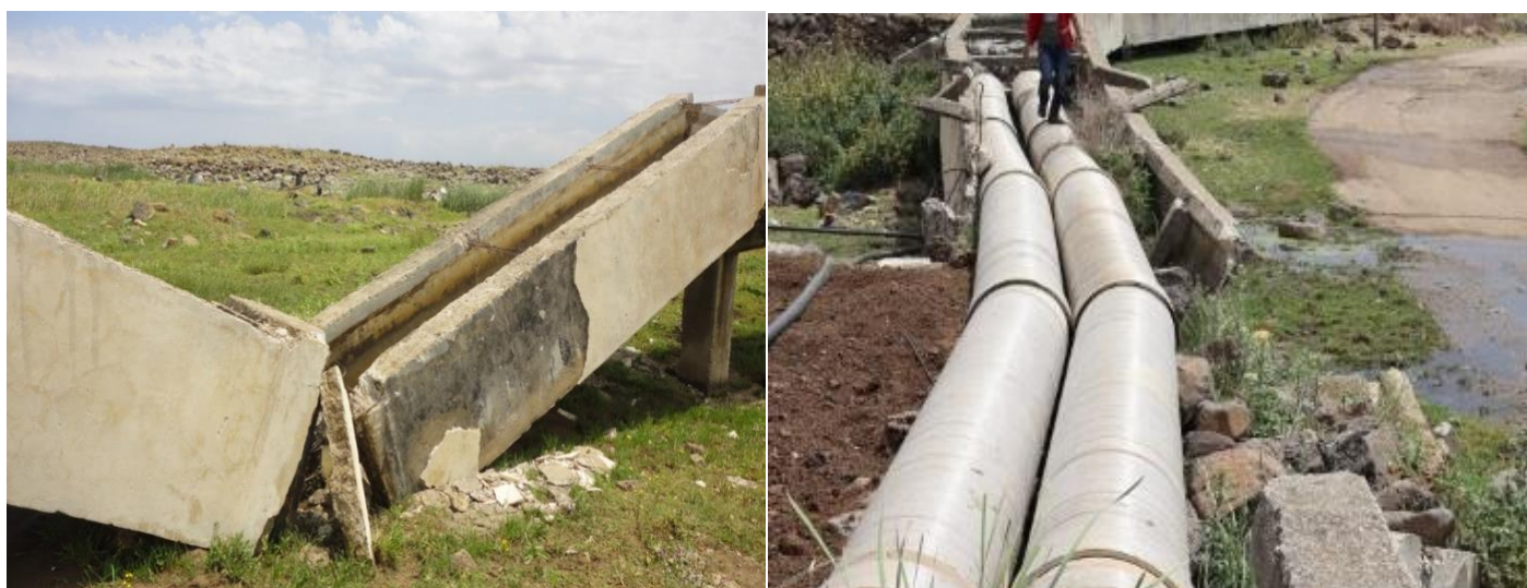
Figure 5: Damages in the main open channel flow within the field irrigation system
