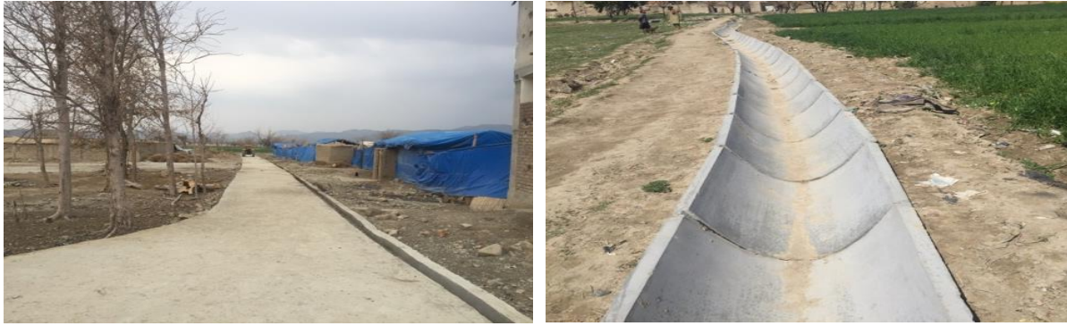
Newly constructed street pavement (left) and irrigation channel (right) in North Waziristan
